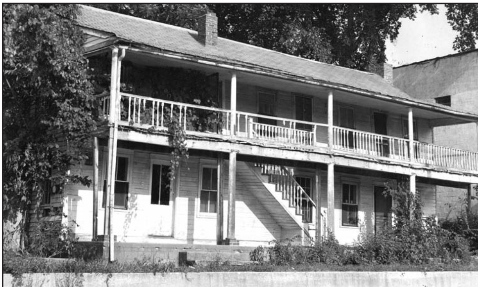
The dilapidated condition of the Old Stagecoach Stop in 1982. It was earmarked for demolition by the City Building Inspector in December of 1982. The owners did not want to restore it. Many concerned citizens expressed the desire to preserve the building. The Old Stagecoach Foundation was formed in June of 1983.
